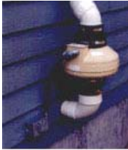
Fan mounted on the outside of a house.
