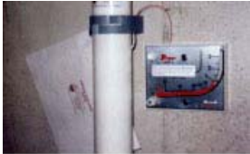
This is an example of a manometer (vacuum monitor) that indicates whether the fan is working properly.
