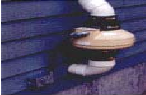
Fan mounted on the outside of a house.
