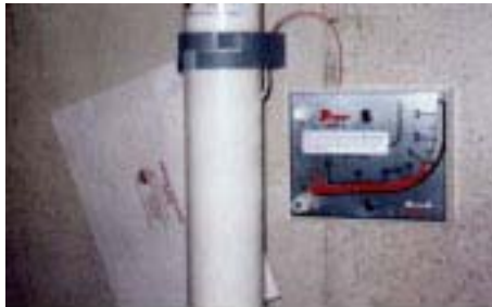
This is an example of a manometer (vacuum monitor) that indicates whether the fan is working properly.
