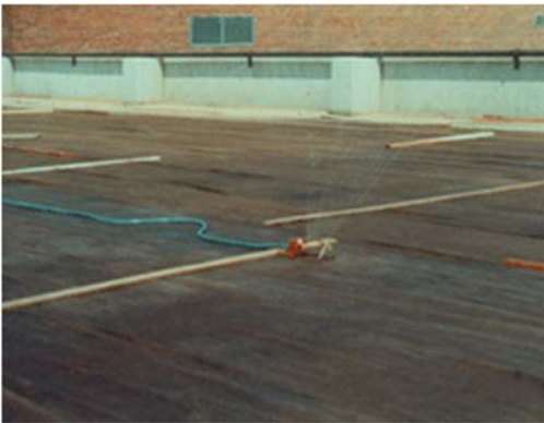
Burlap kept saturated with water is an effective medium for moist-curing concrete.
