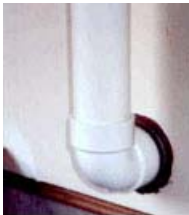
UL listed fire stop assembly in a garage.
